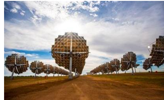
Solar dish technology – world leading efficiency
